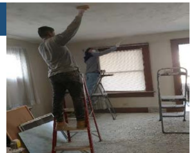
Students volunteered to assist in renovating a home to provide affordable housing in the Akron community.
